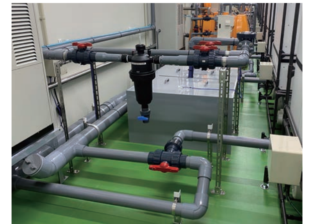
Grow room piping
