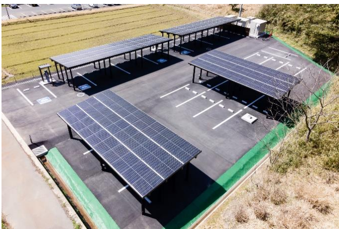
Delivered the “energy earth” for a parking space that can accommodate 20 cars.
